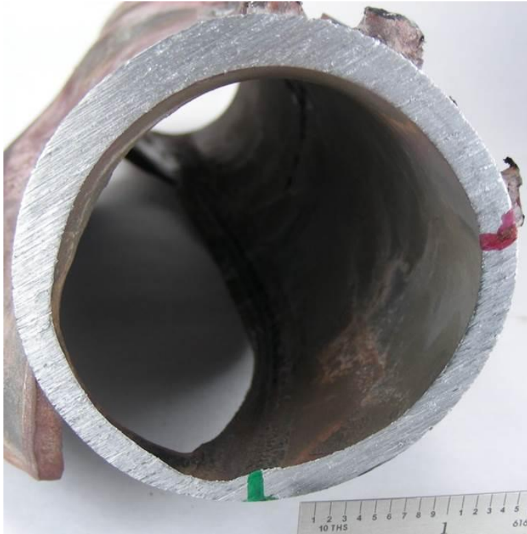
Figure 3. Caustic attack in a cyclone inlet roof tube. The plant commenced load cycling about one year prior to this failure
